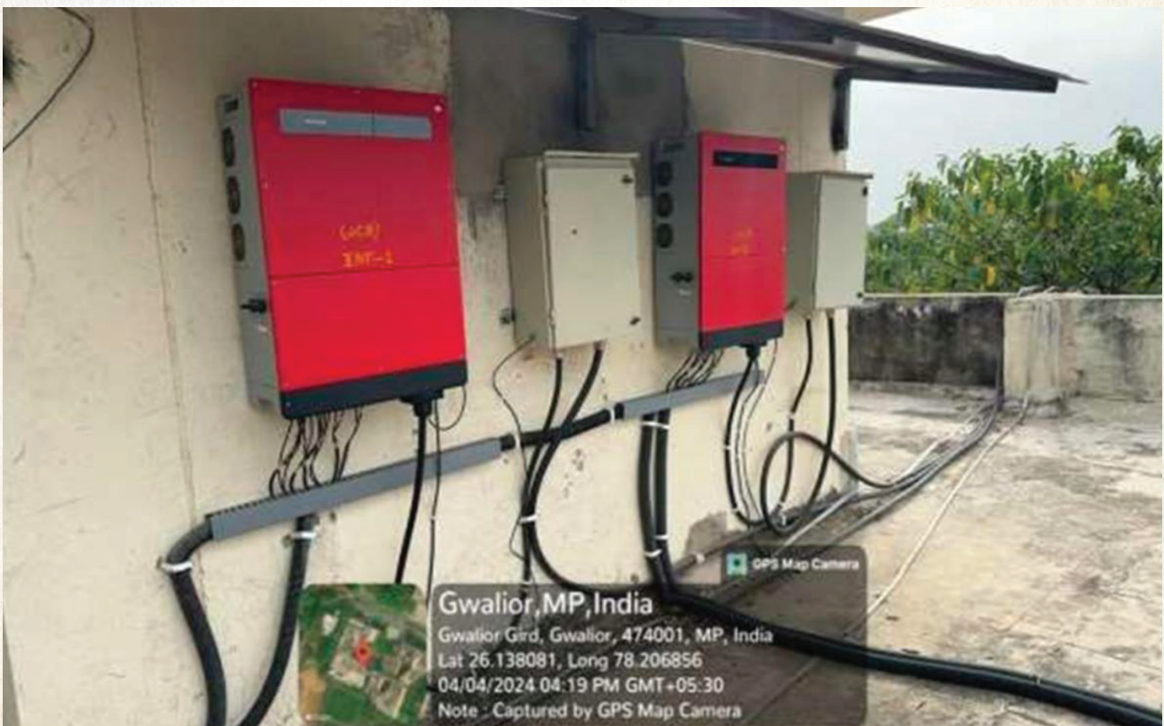
Photos of solar plant & net metering photographs
